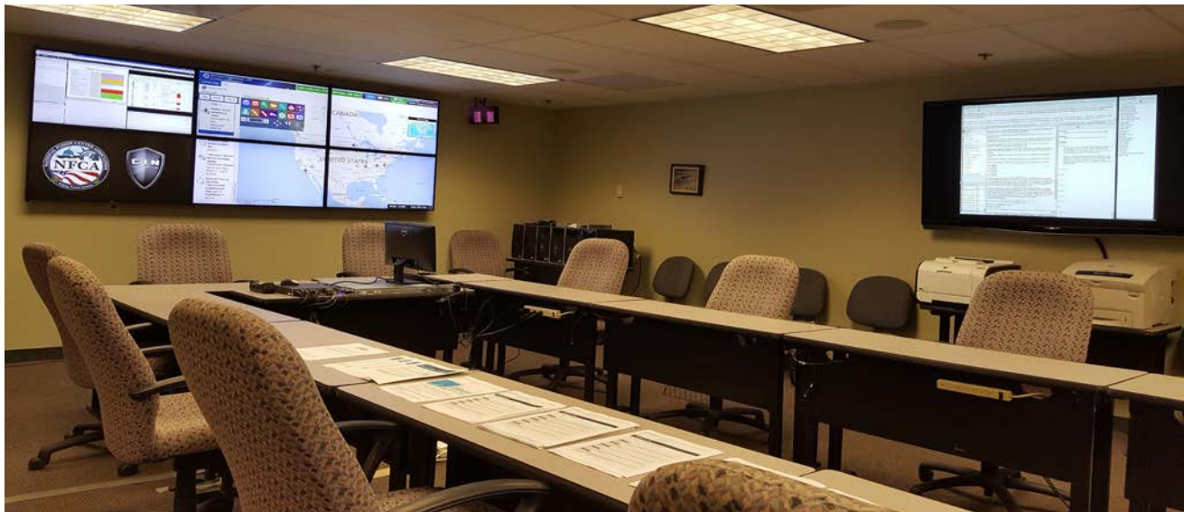
Hiperwall software enables Kansas City Regional TEW Fusion Center to display multiple sources of visual intelligence for decision makers from local, state and federal agencies, including police, fire and the U.S. Department of Homeland Security.
